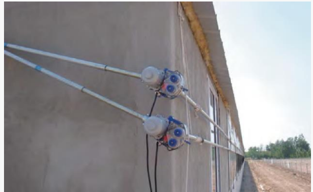
b. Application on Vent System in Livestock
